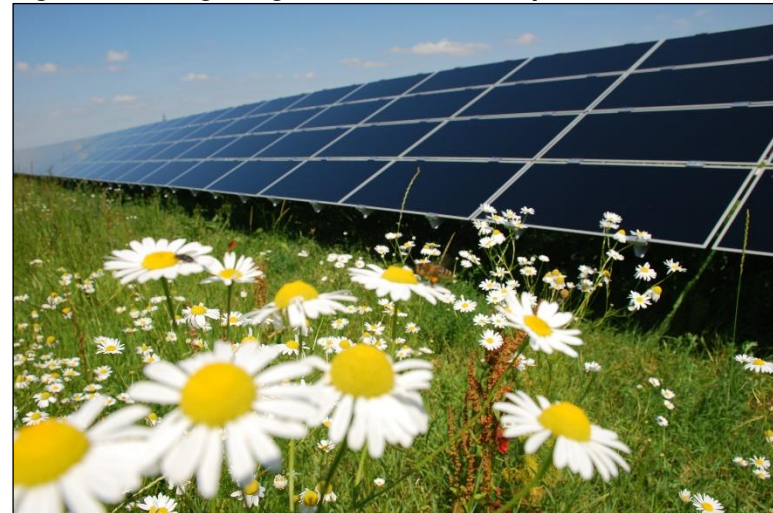
Figure 3.1: Image of ground mounted PV panels
