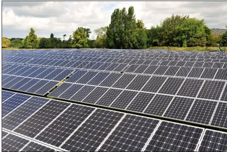
Figure 3.2: Ground mounted PV panels and transformer
